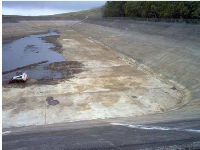
Figure 2: Waikoloa Reservoir No. 1 was partially drained after the 2006 Kiholo Bay Earthquake. It is presently empty and will remain empty until repairs are completed.
