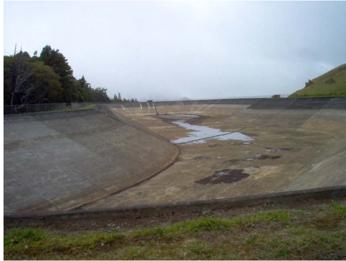
Figure 3: Due to an accumulation of sediment, the reservoir had to be scraped and washed.
